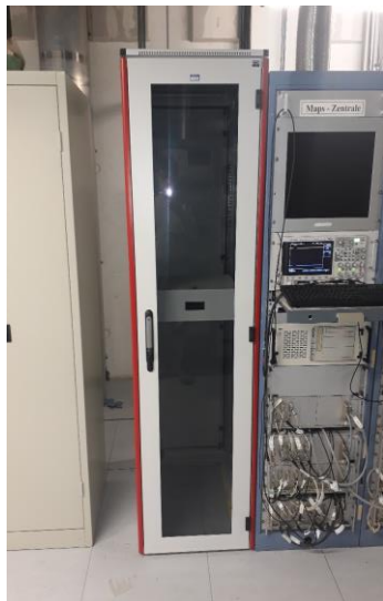
LAN and WR installed
