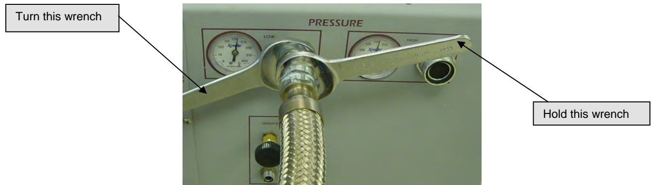
Figure 7-1: Disconnecting flex lines from a compressor package
