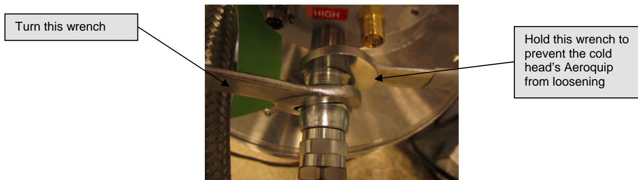
Figure 7-2: Disconnecting flex lines from a cold head
